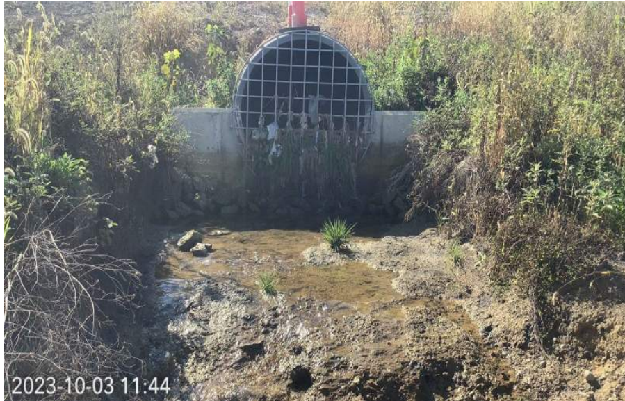
Photo Location 6. View of culvert and manmade upland drainage feature within the Project area. Photograph taken facing southwest.
