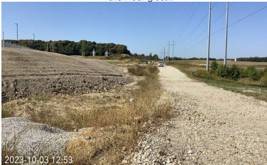
Photo Location 1. Representative view of maintained lawn habitat, existing gravel area, and active construction area within the Project area. Photograph taken facing west.
