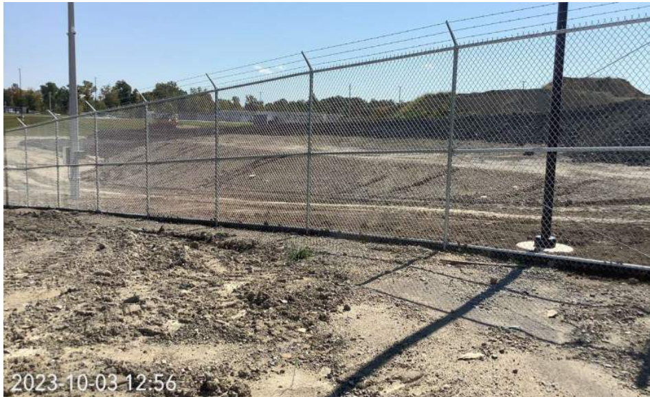
Photo Location 6. Representative view of active construction area within the Project area. Photograph taken facing southeast.
