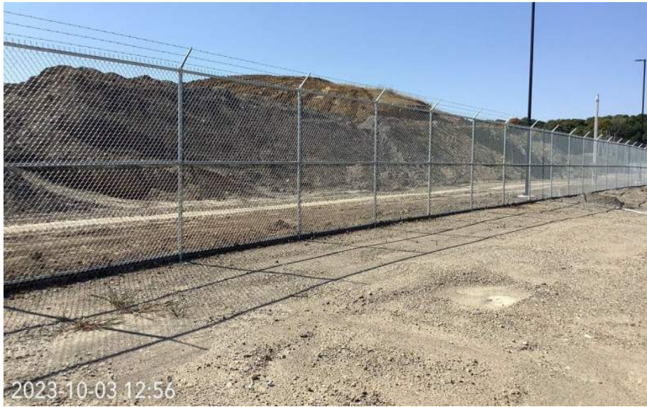
Photo Location 6. Representative view of active construction area within the Project area. Photograph taken facing southwest.
