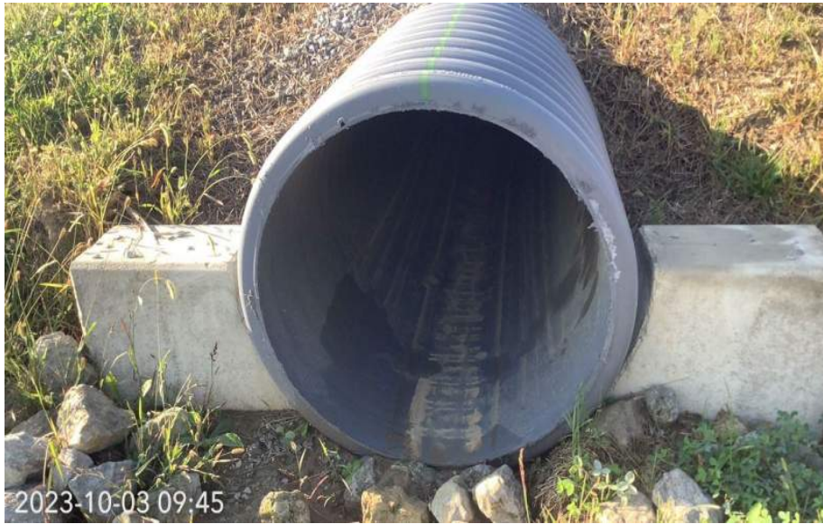
Photo Location 13. View of existing culvert within the project area. Photograph taken facing south.
